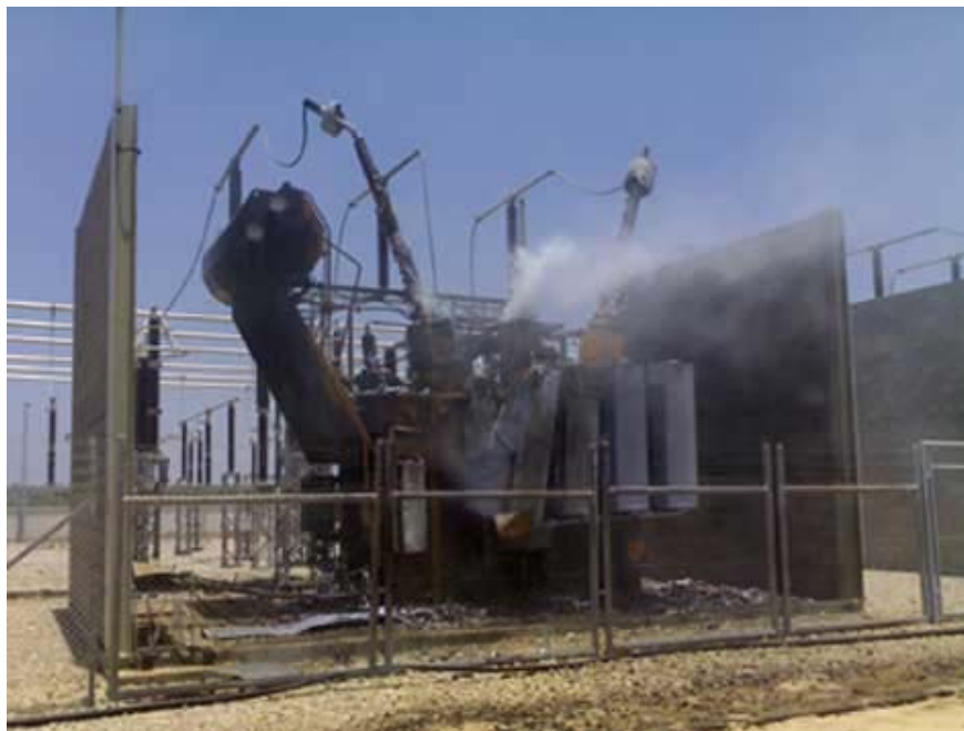
The Gaza electricity generation facility which was destroyed by an IOF air strike on 26 June 2006.
